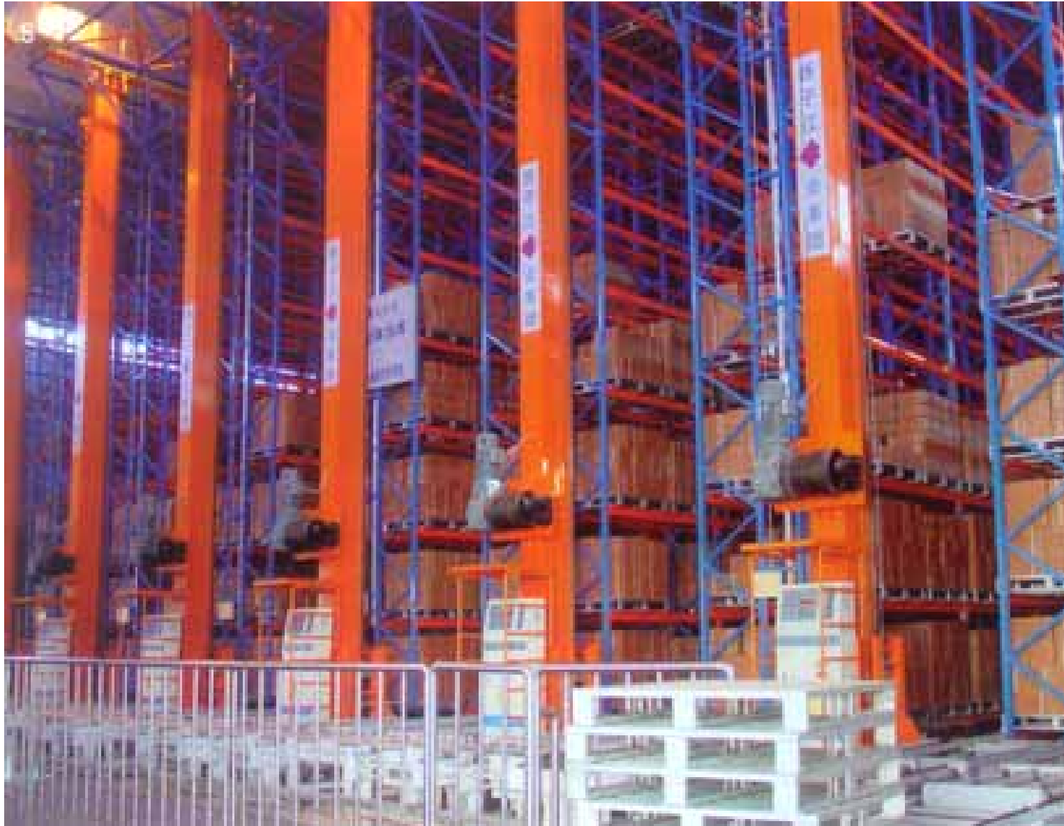
Automated high-rise warehouse, Yangzi-River Pharmacy Group
