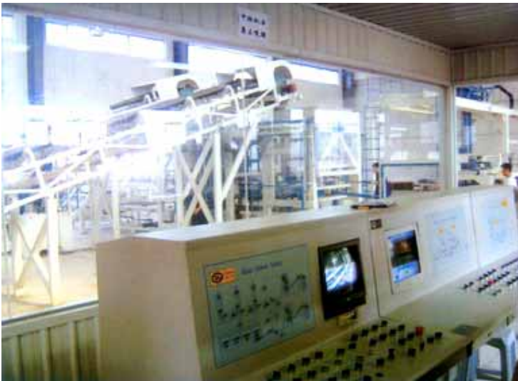
Central control room
