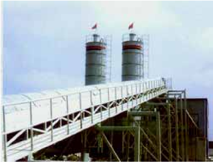
Material batching system
