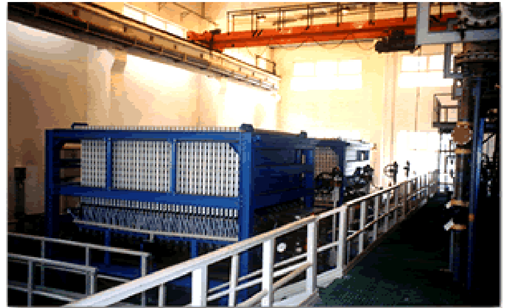
28,000 TPY potassium hydroxide project of Jiangsu Guangming Chemical Co., Ltd. Jiangsu, China (2002)
