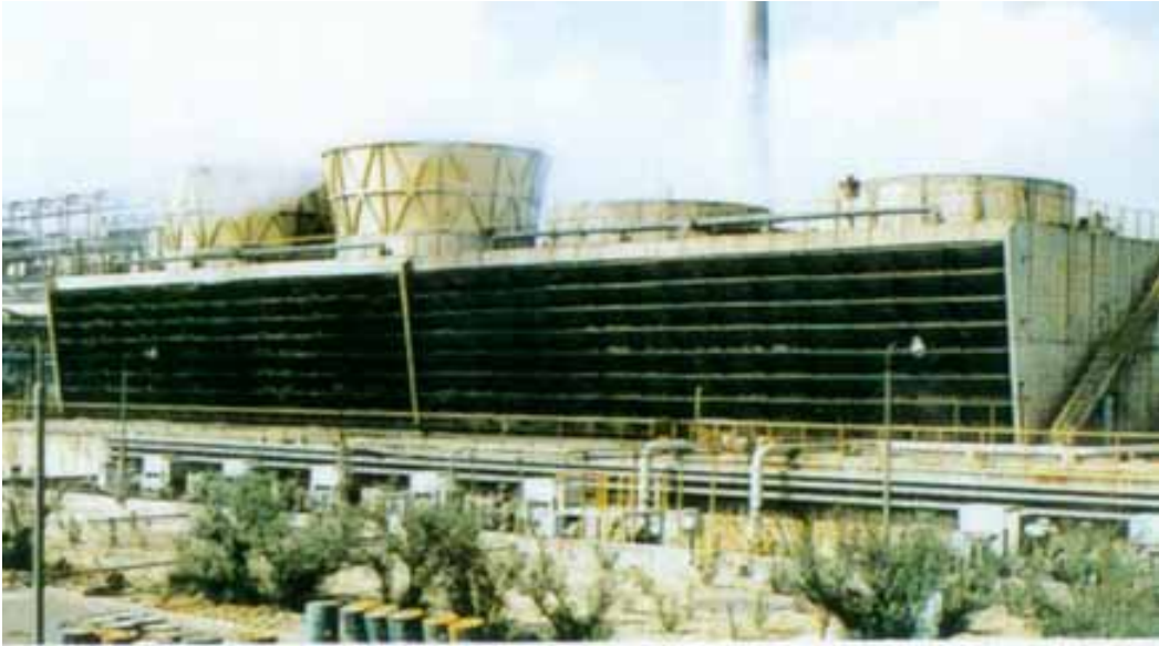
Clean water recycling system
