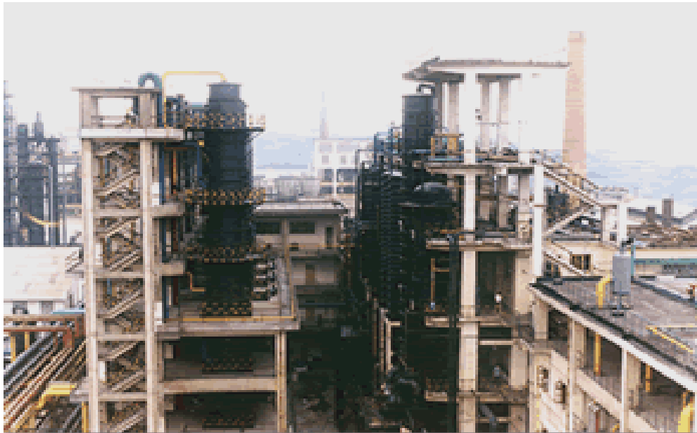
285,000 TPY soda ash & ammonium chloride co-production project of Honghe Chemical Plant, Sichuan, China (1989)
