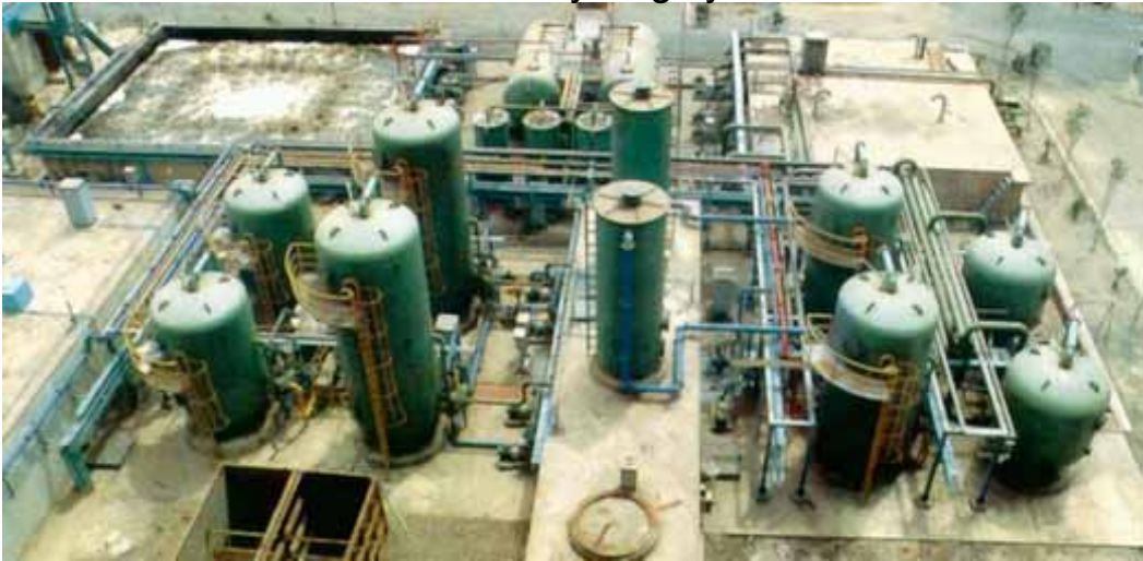
Pure water treatment system
