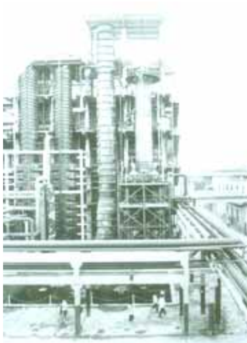
Natural circulation outer cooling carbonization tower
