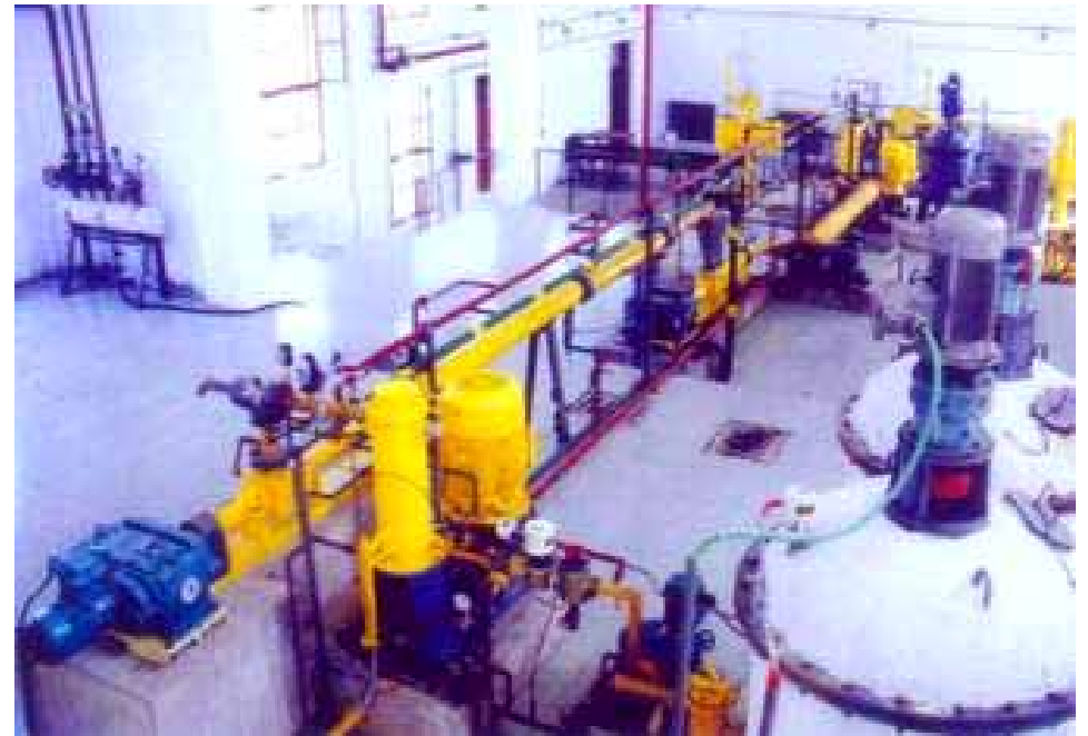
Emulsified explosive production line, Fendou Chemical Plant, Heilongjiang
