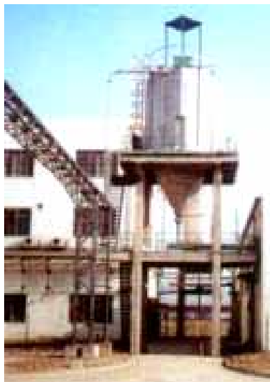
Pneumatic conveying system
