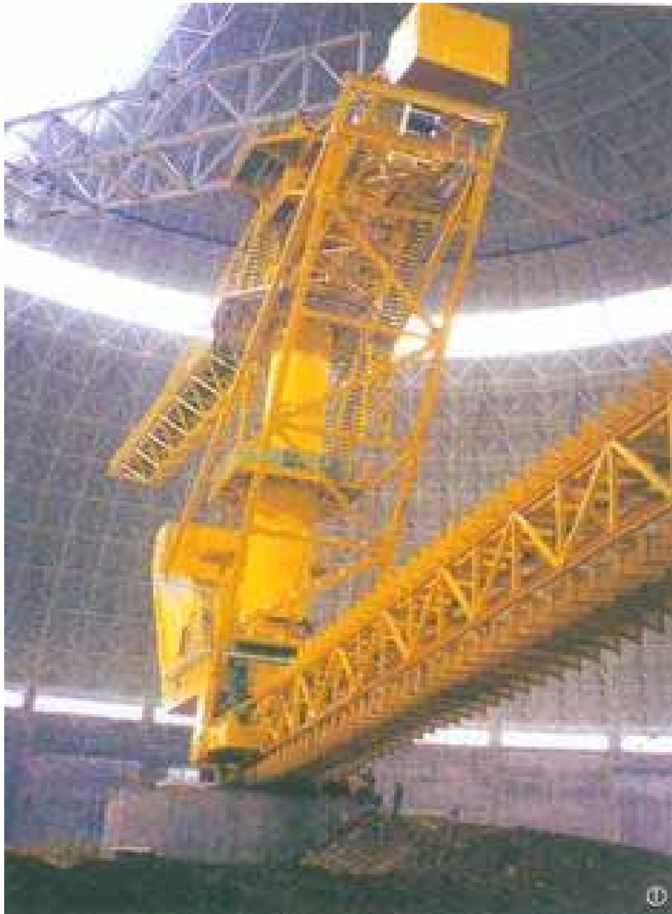
Circular storage yard, top stocking and lateral reclaiming
