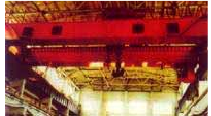
General-purpose overhead traveling crane
