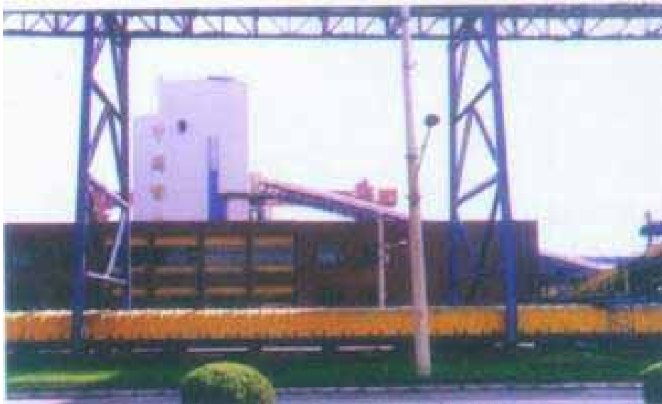
Sampling and sample preparation system for coal terminal
