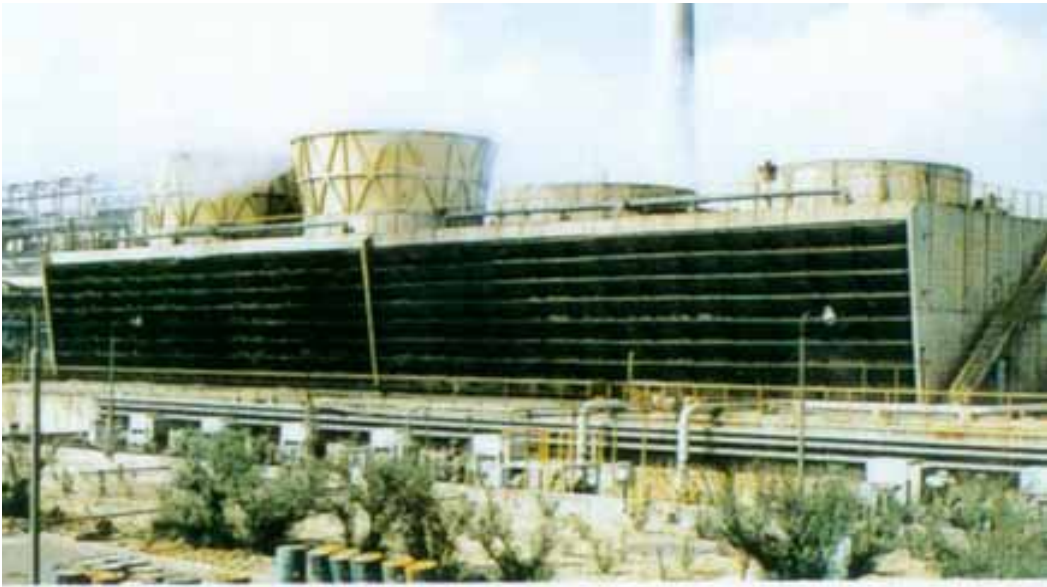
Clean water recycling system
