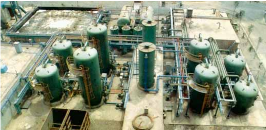
Pure water treatment system
