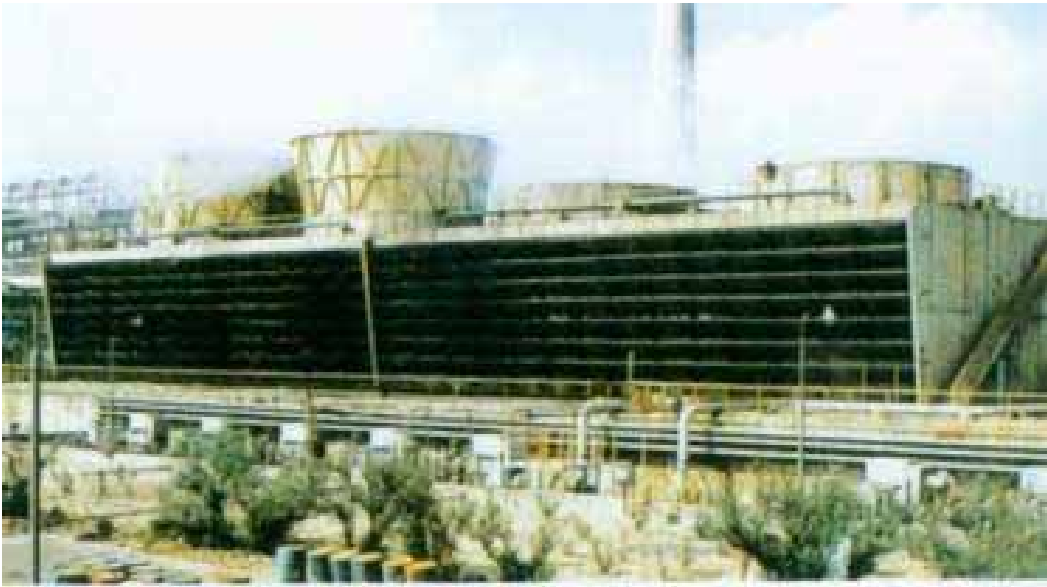
Clean water recycling system
