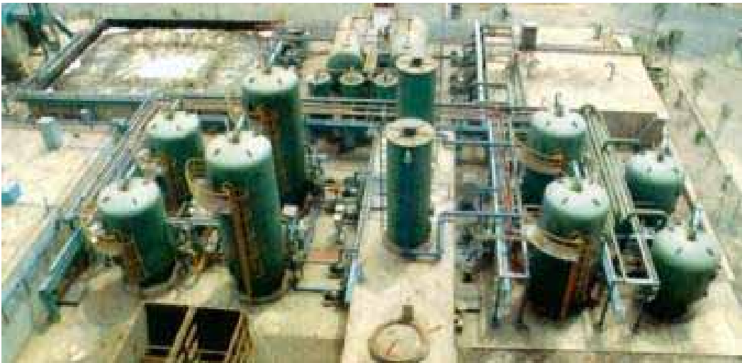
Pure water treatment system
