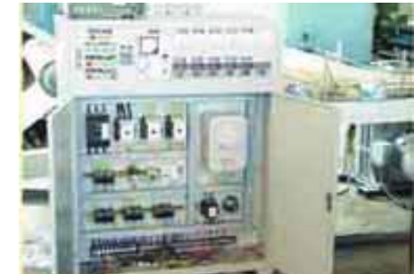
Electrical control cabinet
