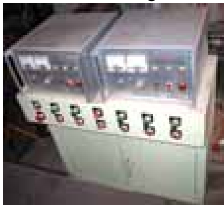
Control at the rear section
