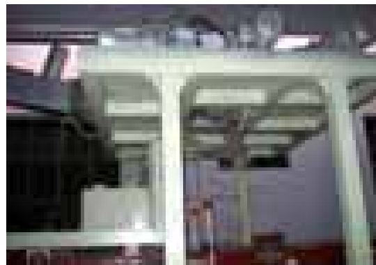
Vacuum pump and heating
