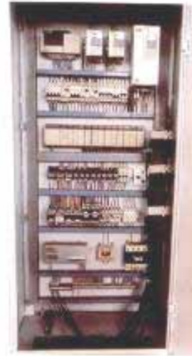
Electric Control System
