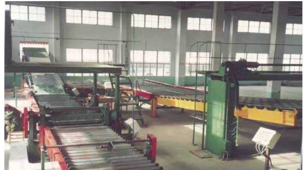
Conveyer roller, cutter, and distributor, etc
