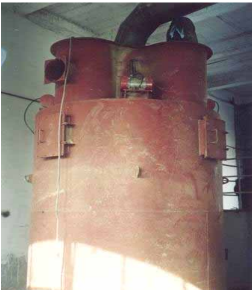
Electrical dust collection for fluidized kiln
